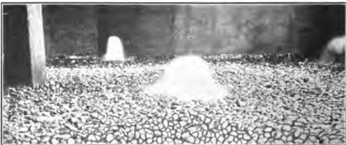
Stone filter beds in a sewage disposal plant.
